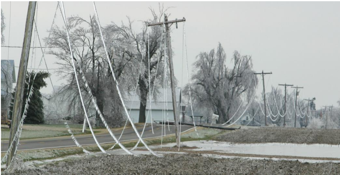
Figure 3: Severe weather conditions (e.g. an ice storm in figure) are triggering power grid failure.
